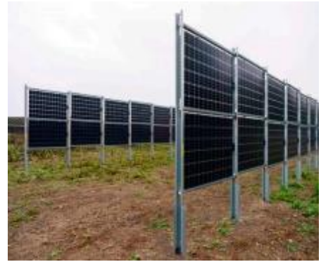
Figure 5.1. Vertical PV (Source: Next2Sun)
