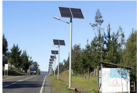
Figure 4.7. An example of PV street lighting
