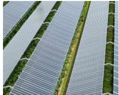
Figure 5.2. Elevated PV without tracking (source: Baywa)
