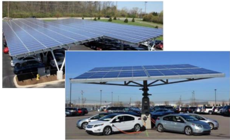
Figure 4.4. Solar carports on parking lots
